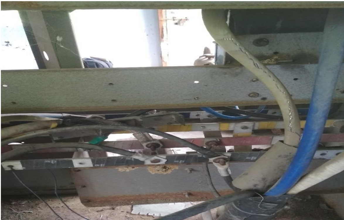
Damaged Power Cable Found in panel of Incomer Transformer
